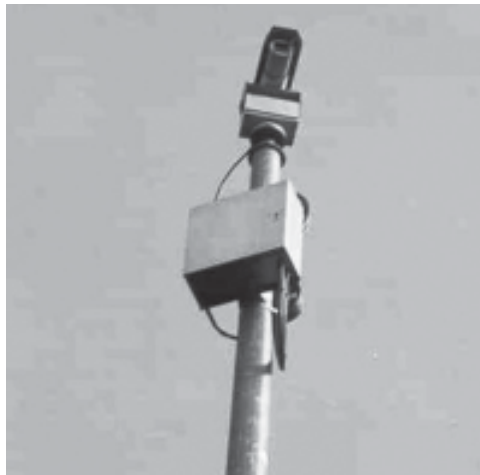
(ဋ) CCTV camera using microwave transmission
